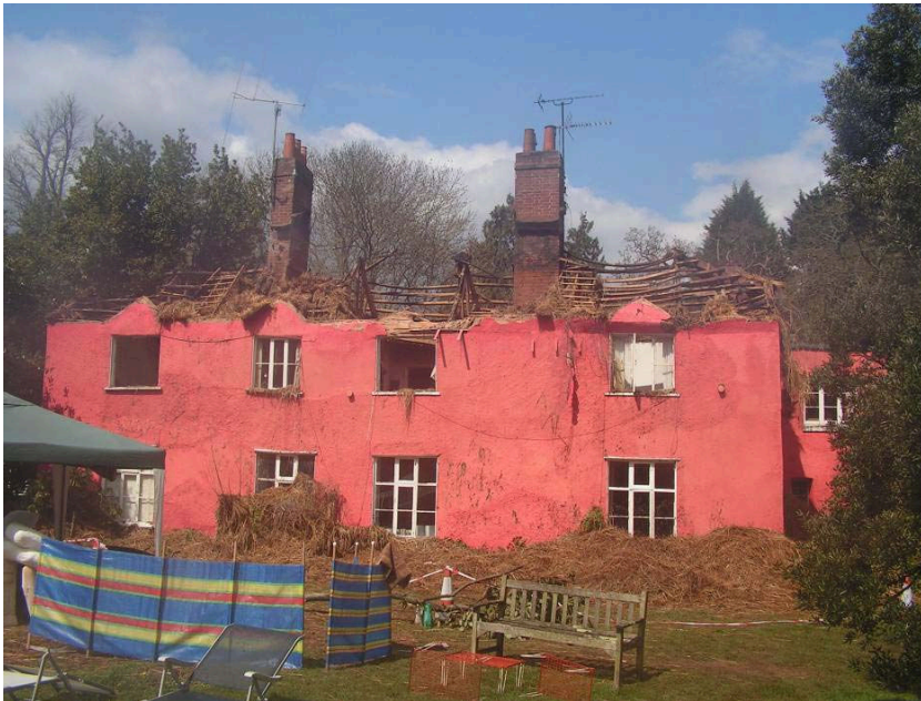
Holmbush after the fire, April 2012
